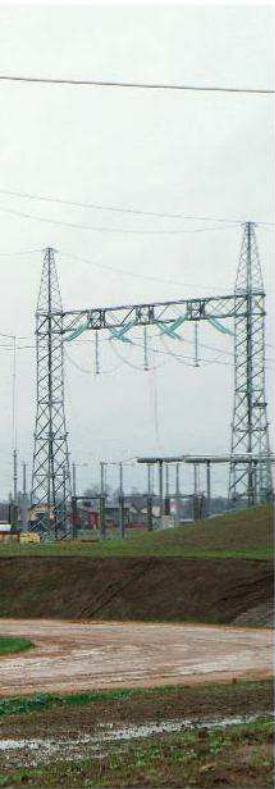
High-voltage power lines, like these linking Poland and Lithuania, counter renewables' reliability problem
